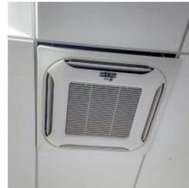
Ceiling Heat Pump
